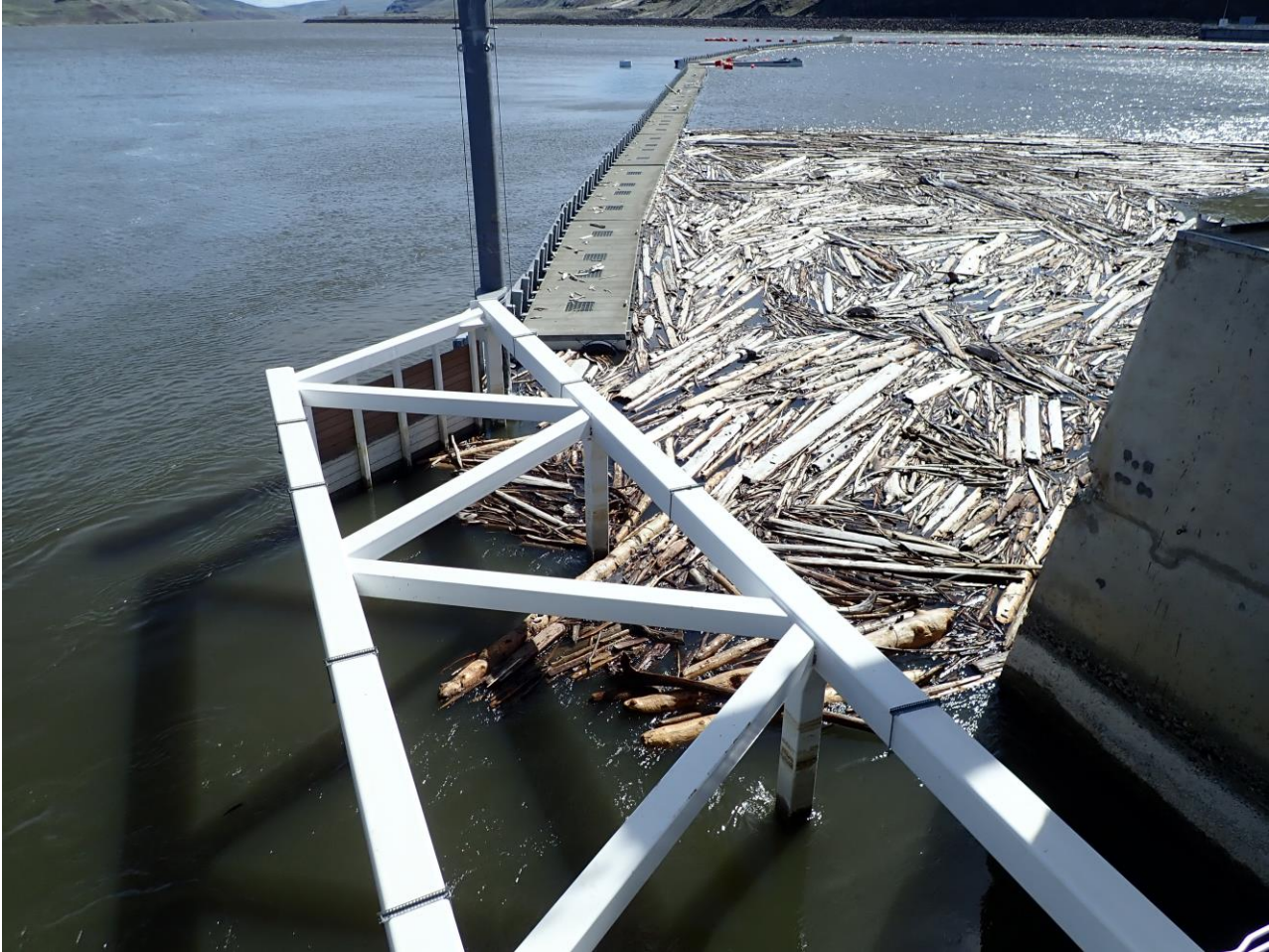
Image 1: Debris caught near Unit 6 and adjustable spillway weir on April 10, 2019.
